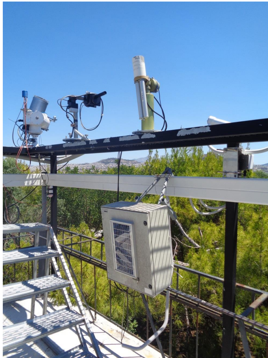
Bad direction of Solar Panel #440 ATHENS_NOA
